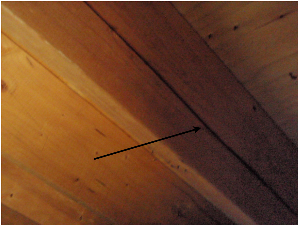
Photo 2. This is the cracked attic rafter.
