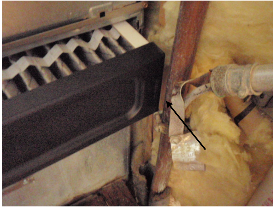
Photo 3. The main water supply pipe is blocking the furnace filter.
