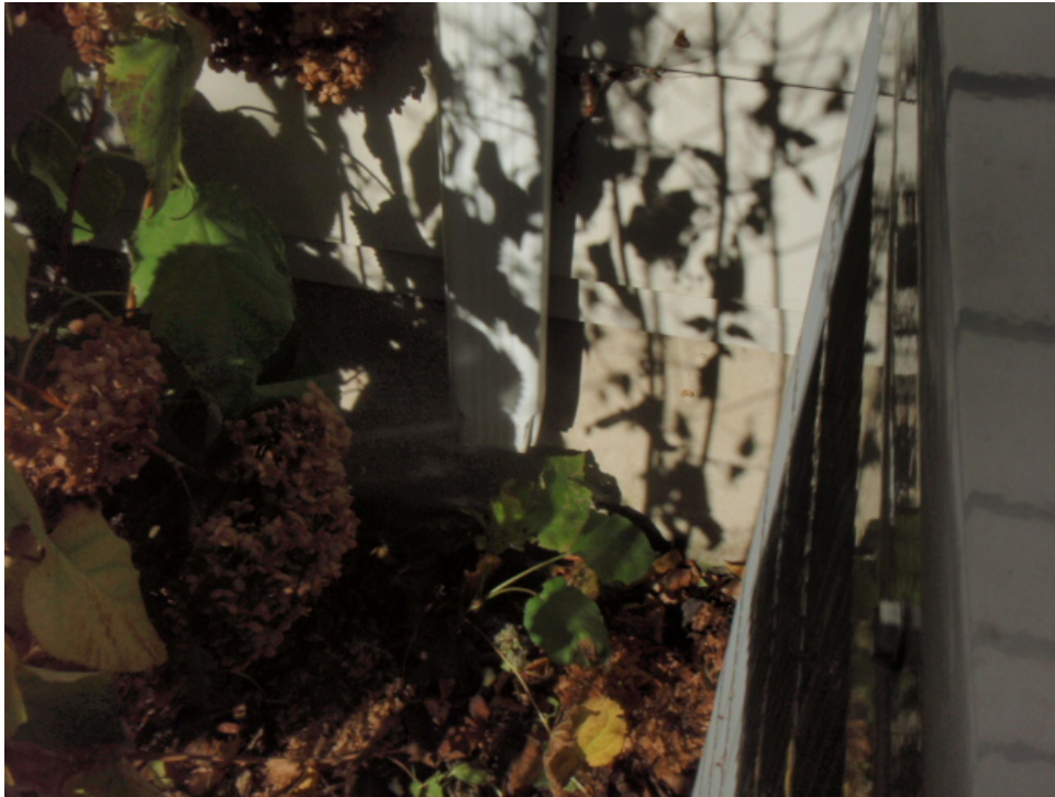
Photo 5. The downspout is disconnected and discharging alongside the foundation. This may cause basement flooding.
