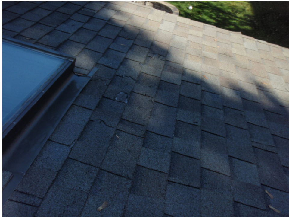
Photo 6. There are numerous worn shingles on the south elevation. This may cause a roof leak.
