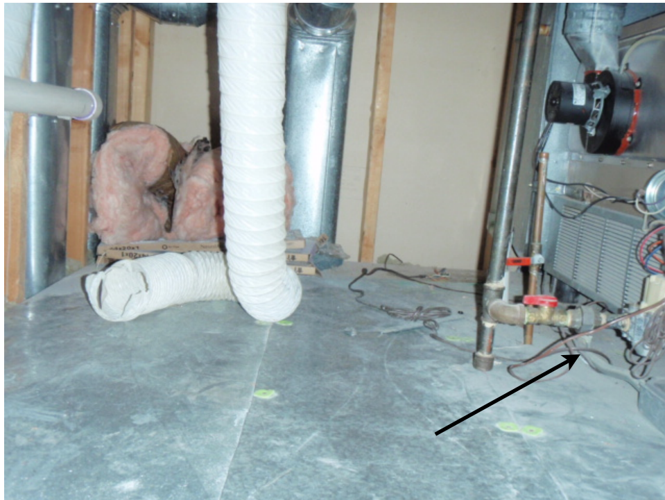
Photo 4. There is no overflow pan under the second floor furnace. This may cause a water leak in the ceiling below.
